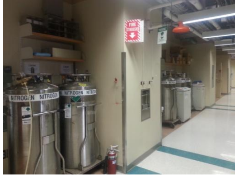
Multiple liquid nitrogen tanks in a linear equipment room, no oxygen sensor is present.
