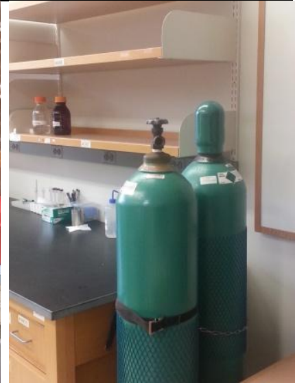
No protective gas cap.
