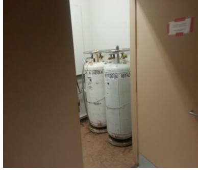
Liquid nitrogen being stored and dispensed in a small storage room with no oxygen sensor.
