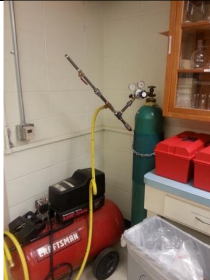
Modified tank using inappropriate plumbing materials with Teflon tape.
